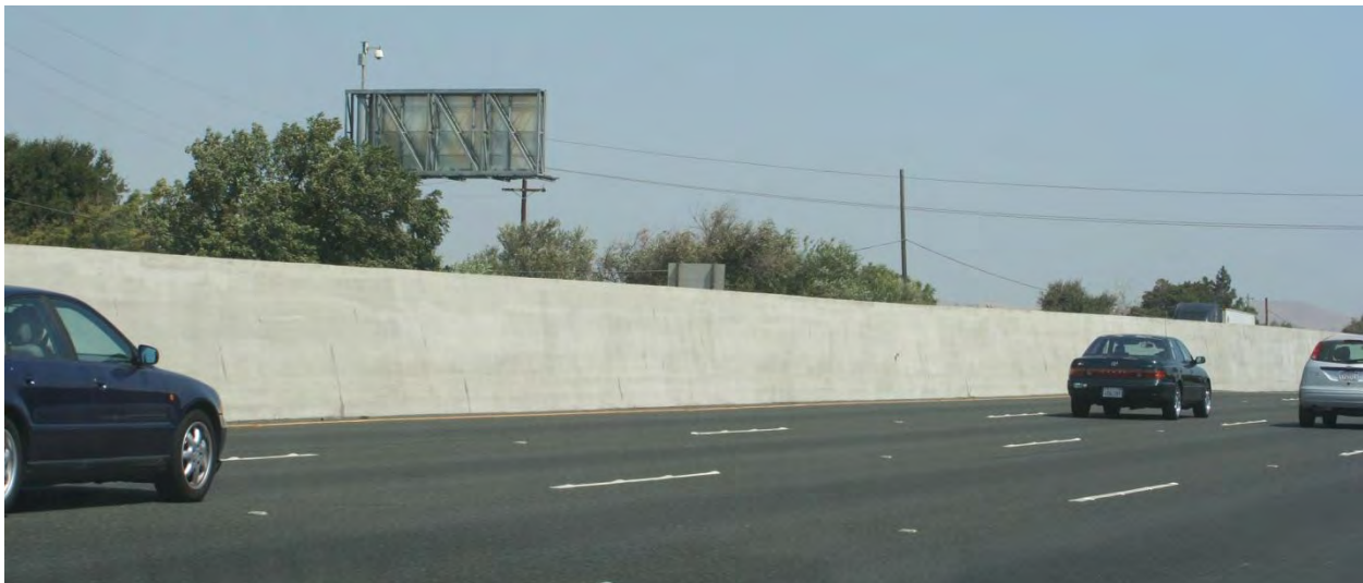
Median Divider Treatment – Structure is taller than normal due to elevated roadway in the opposite direction.
